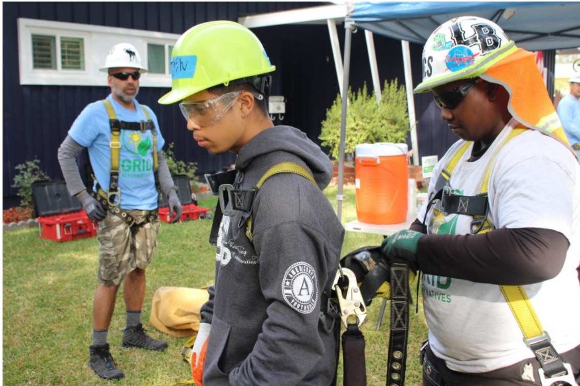
A man gets fit with a harness before helping to install solar panels on the roof of a low-income family's home in Santa Ana. (Courtesy of Danny Hom)
