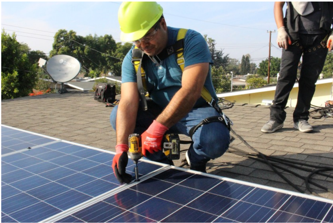
A man installs solar panels on the home of a low-income family in Santa Ana. (Courtesy of Danny Horn)
